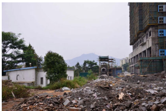
Figure 36: There are still a lot of construction sites in Guangming new town without any people.
