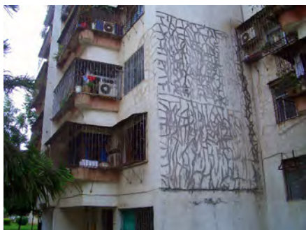
Deterioration (Source: bbs.szhome.com)
