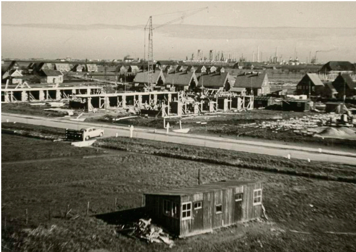
Plan West, construction works for the new Zeeheldenbuurt (1957) Source: municipality of Nissewaard
