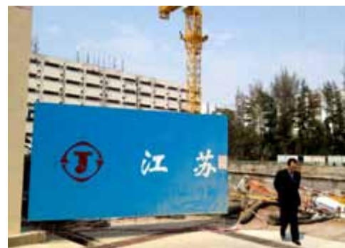
Construction site where in the near future a new addition to Shenzhen's endless number a high-rise gated complex will be built. Construction sites like these are seen all over Shenzhen.
