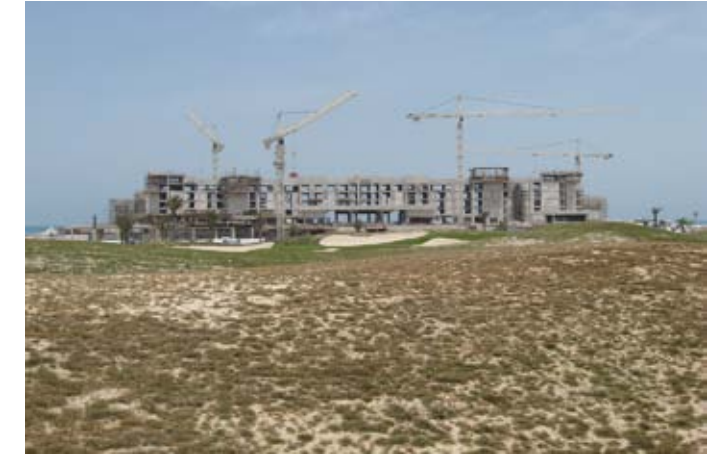
Developed by Abu Dhabi National Hotels (ADNH), The Park Hyatt Abu Dhabi Hotel is currently under construction next to the Saadiyat Island Golf Course. The hotel will have 270 guest rooms, and fifteen private villas, 2010.
