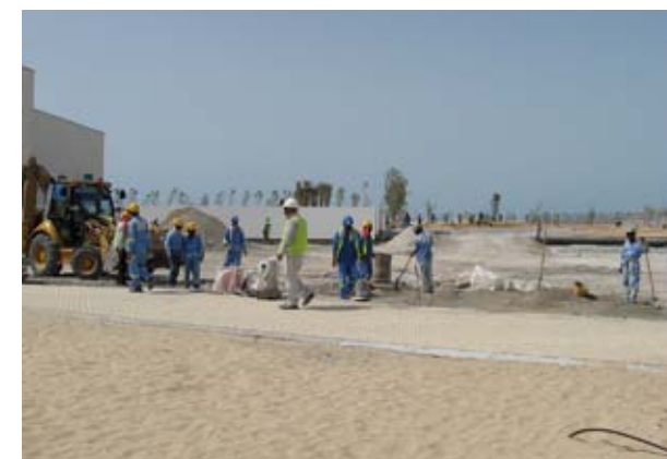
Construction workers make headway on the 15,000 m 2 Manarat Al Saadiyat exhibition space, 2010.
