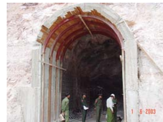
Military officials inspect the entrance to the underground Taunggyi command post during construction.
